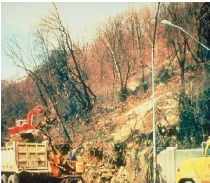
A highway crew removes material along the Columbia Parkway in Cincinnati, Ohio. Leaning trees are an important indicator for unstable ground. Photography by Bob Fleming, USGS.
